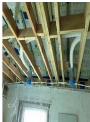
Air ducts in ceilings
